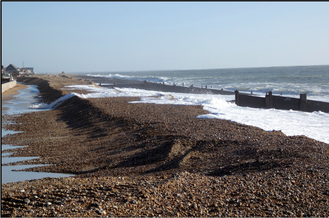
Overtopping at Eastoke 25.11.22 following the rebuild
