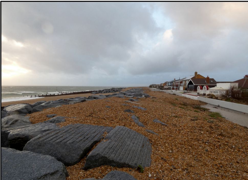
Granite Blocks in front of Creek Road overtopped
