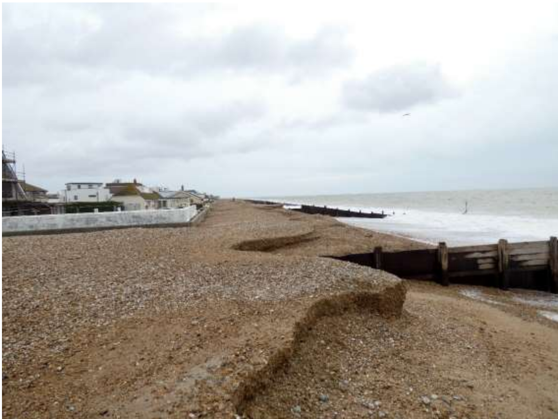
Pic 3: Showing the erosion at Eastoke 2 weeks after Pic 2 was taken
